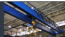
Over Head Crane
